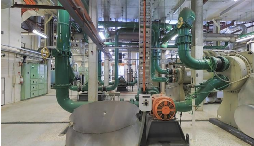
Large Mechanical Plant
